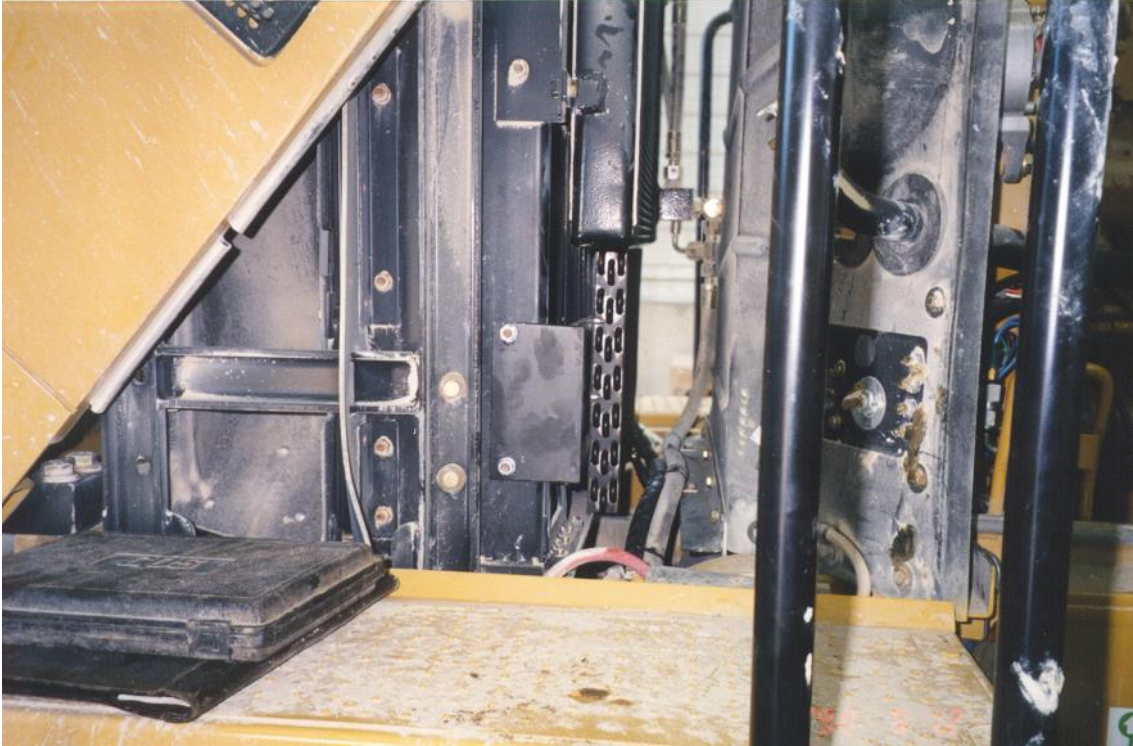
Condenser as viewed from right side.
