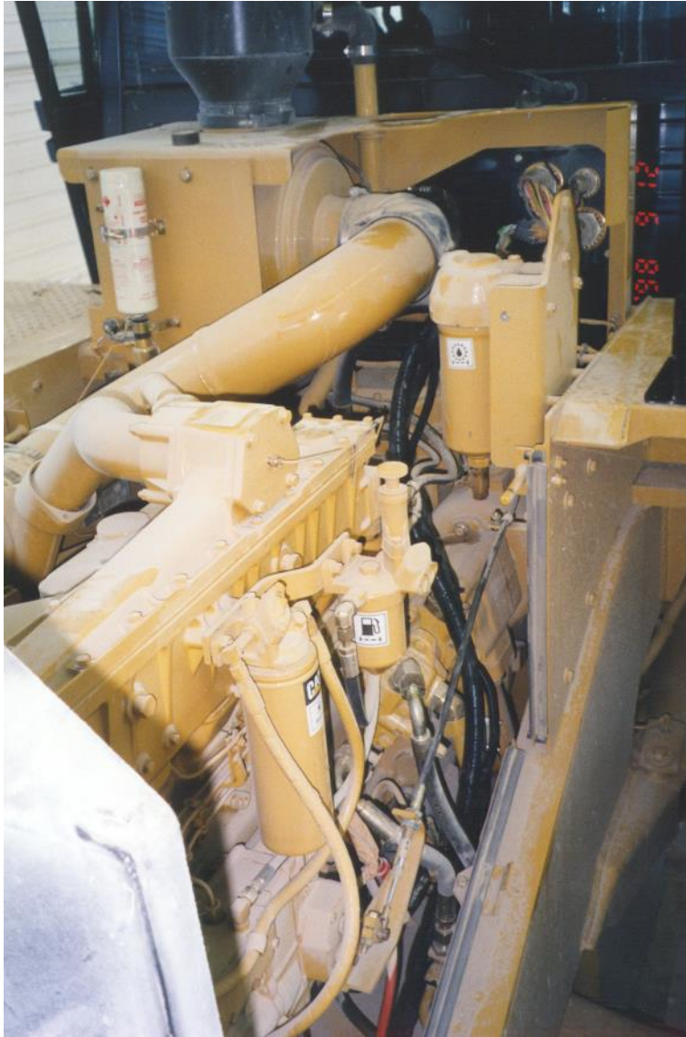
Hose routing through engine compartment.
